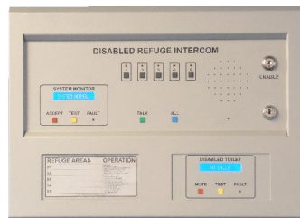
Fig 7:10 Remote Indicator Panel Kit Mounted in Compact Disabled Refuge EVC Master Station
